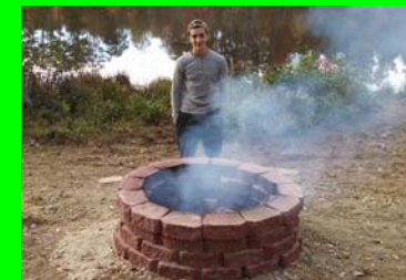
Fire pit, retaining wall - American Legion Post 116
