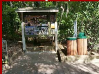
Retention Wall – Hemlock Bluffs Nature Preserve
