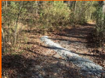
Trail erosion channels – Northern High School
